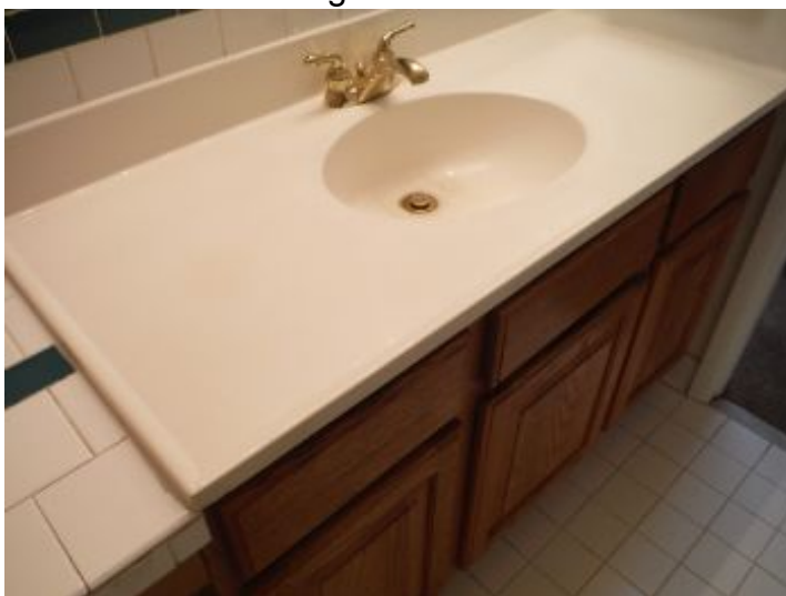
Counter top loose
