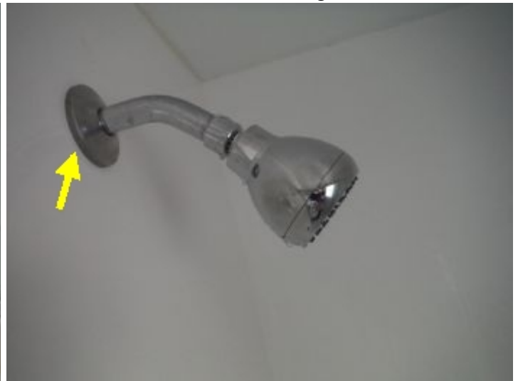
Loose shower mast
