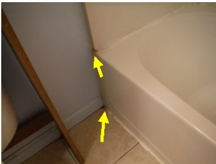
Failed or missing sealant Basement bath
