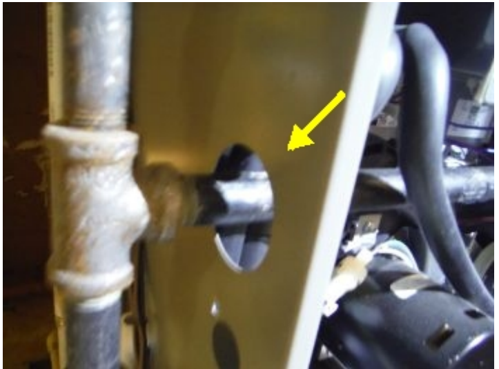
Failed or Missing sealant.
