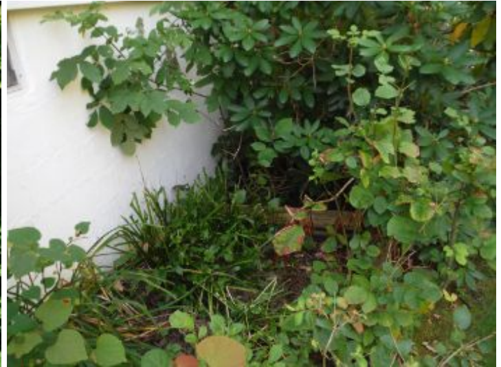
Vegetation closer than recommended.
