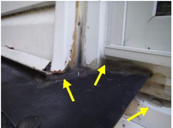
Failed or Missing sealant
