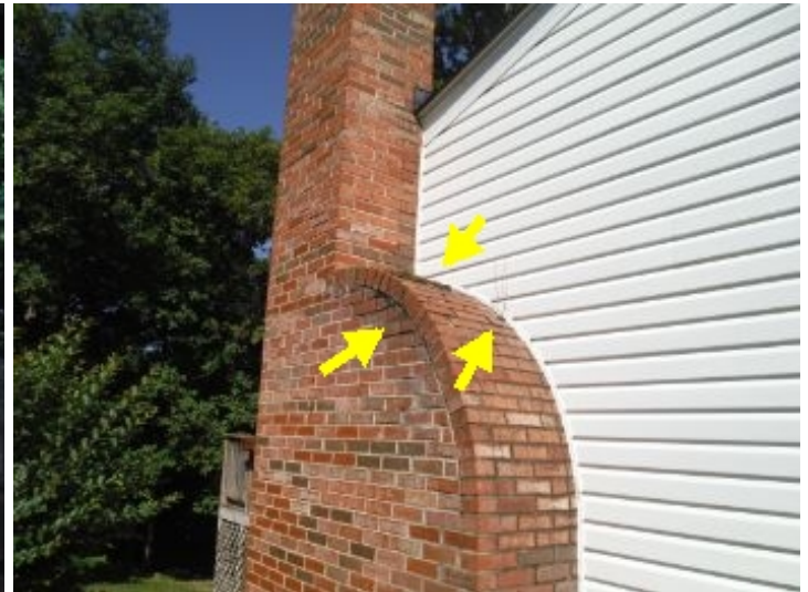
Brick and/or Mortar deterioration/ Moss growth
