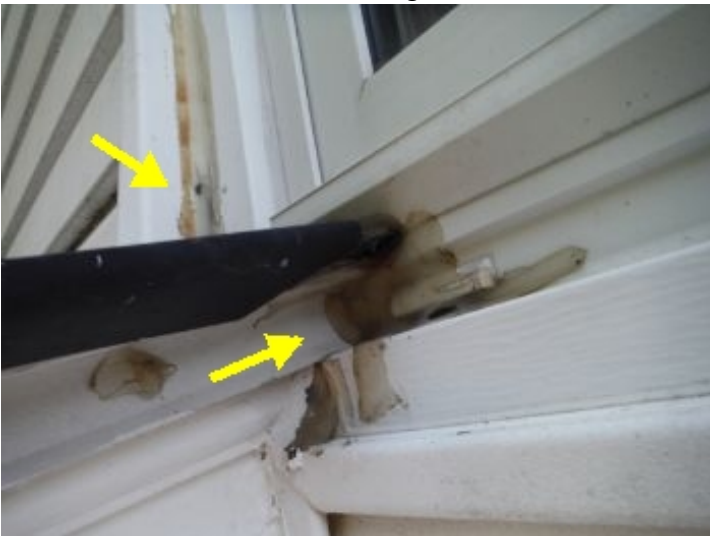
Failed or Missing sealant
