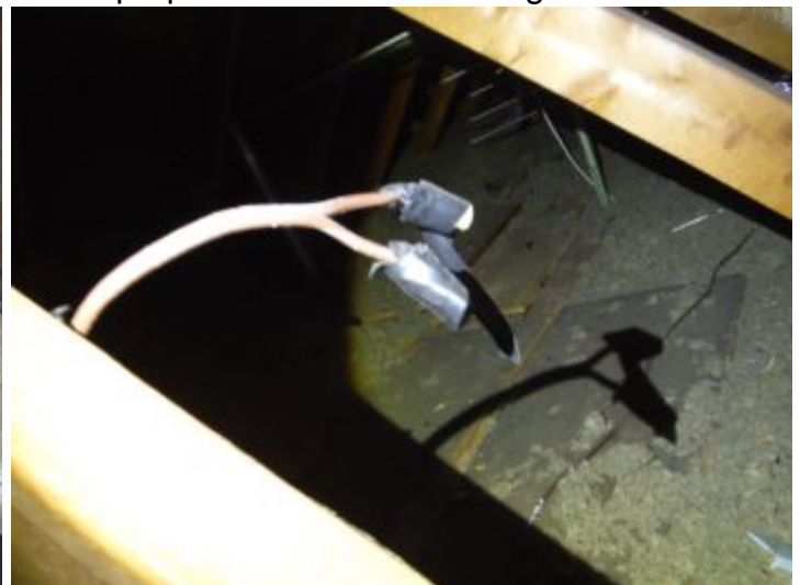
Missing Junction box.
