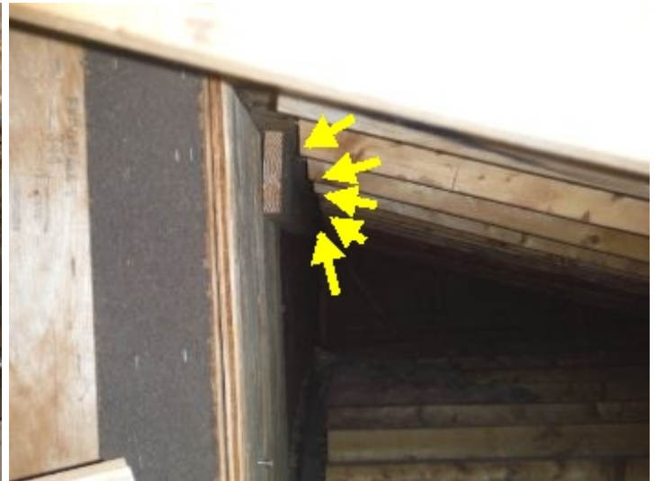
Improper connection. Missing connectors
