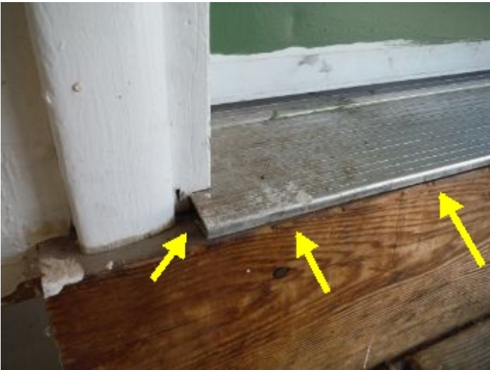
Failed or missing sealant
