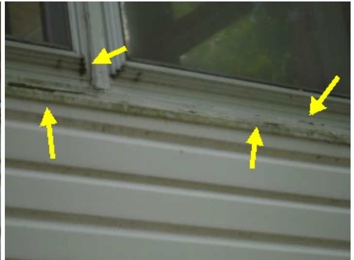
Damaged window frame.
