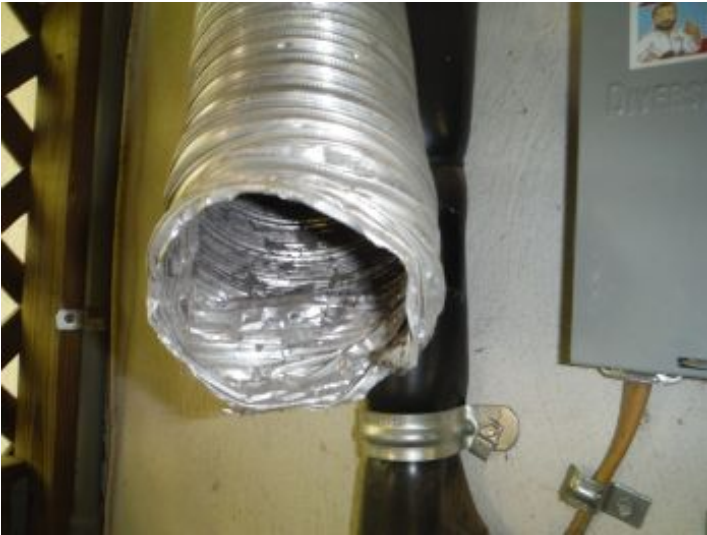
Dryer vent not secure/ missing screen
