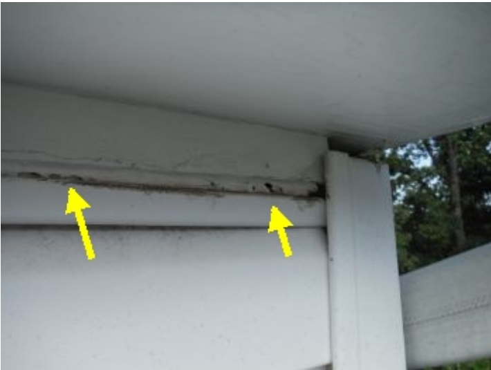
Failed or Missing sealant
