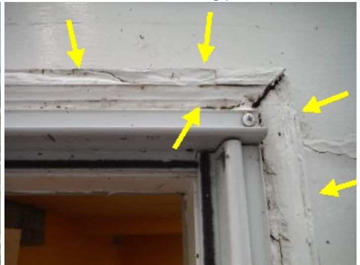
Wood deterioration noted.
