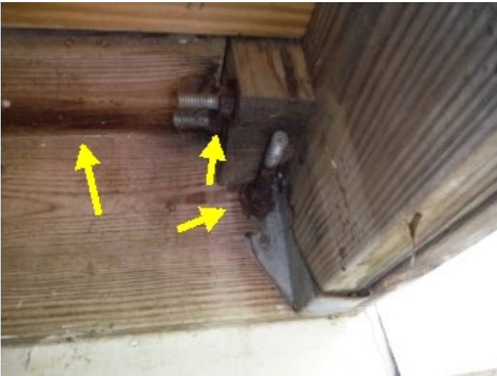
Ledger board flashing not visible/rusted fasteners
