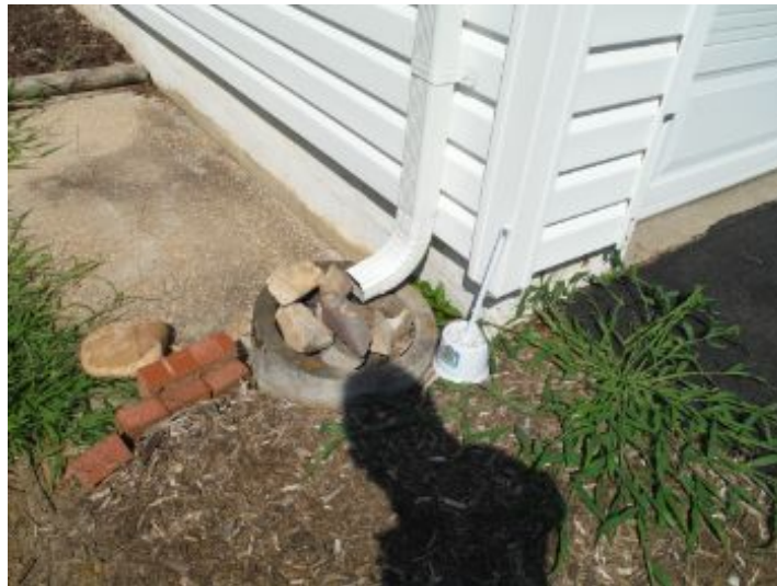
Downspouts Extension missing; recommend installation.
