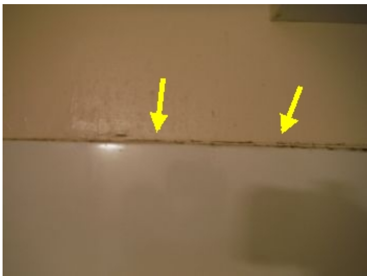
Failed or missing sealant Basement bath
