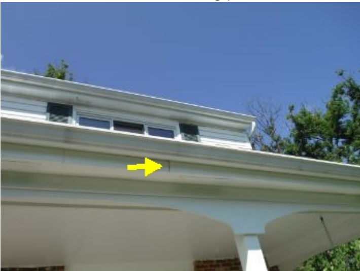
Failed or Missing sealant
