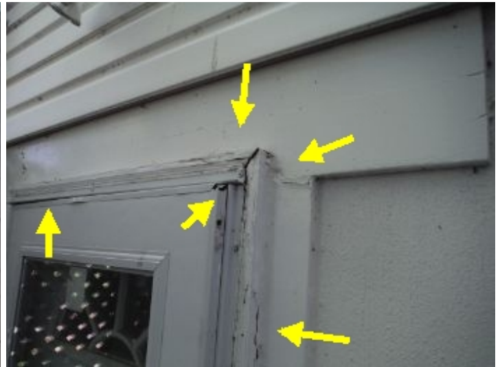
Wood deterioration noted.
