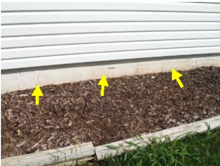
Crack visible in foundation Parging
