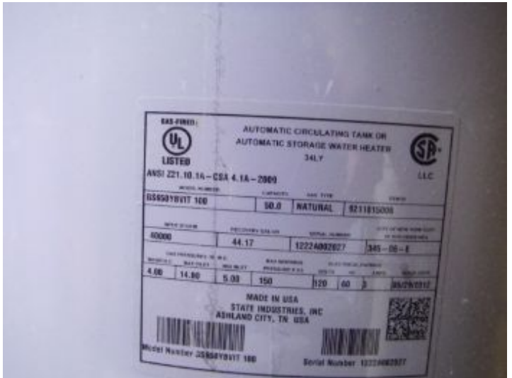
Data Tag Water Heater
