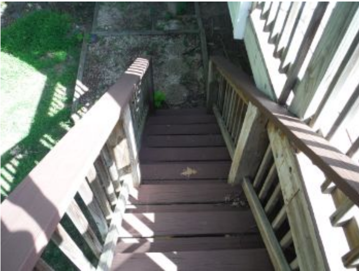
Handrail not graspable
