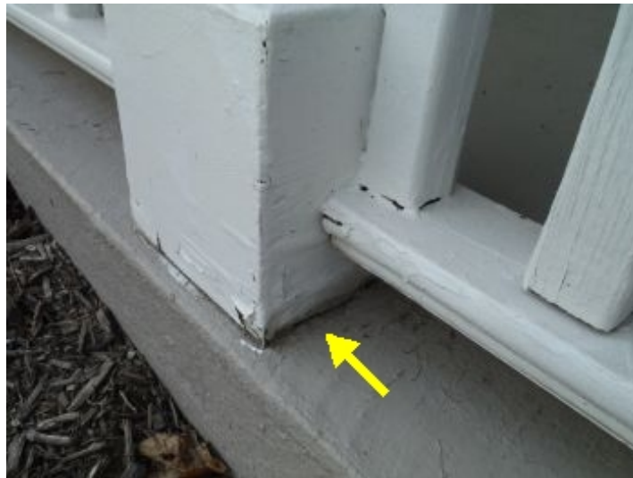
Wood deterioration noted. Have repaired as necessary. Front Porch
