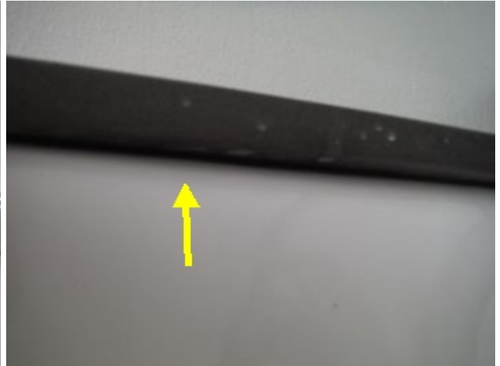
Failed and/or Missing sealant
