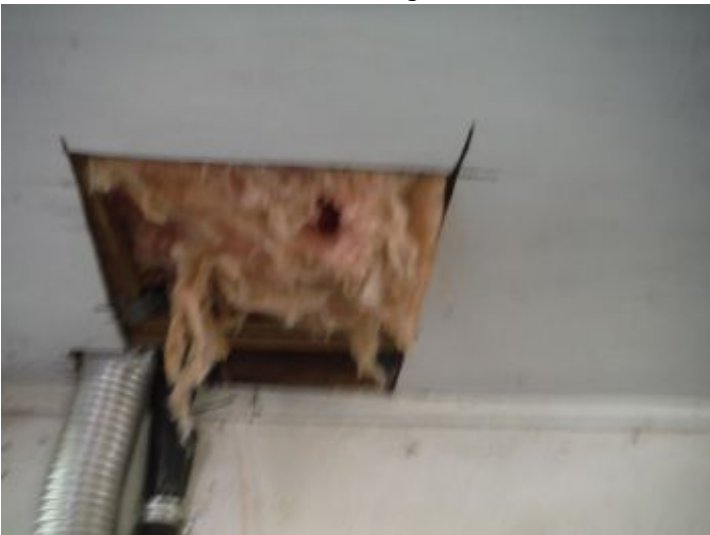
Exposed insulation/ missing siding
