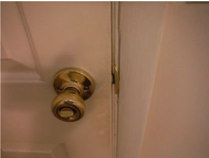
Misaligned strike plate.
