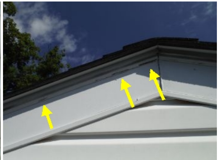
Failed or missing paint
