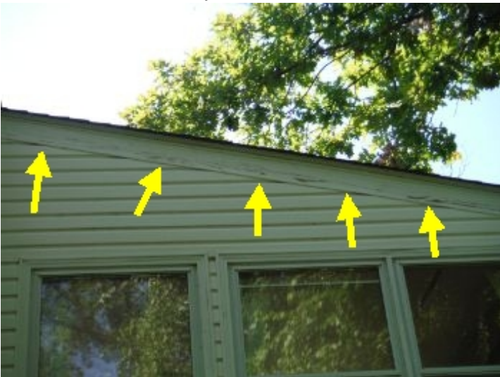
Failed or missing paint
