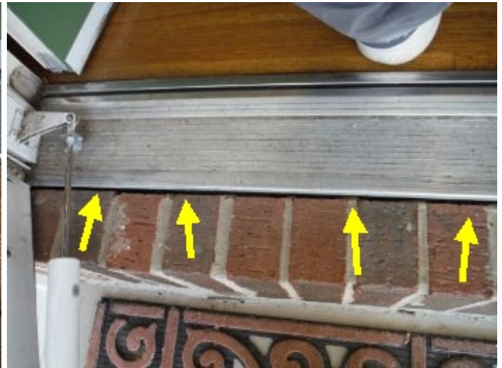
Failed or missing sealant
