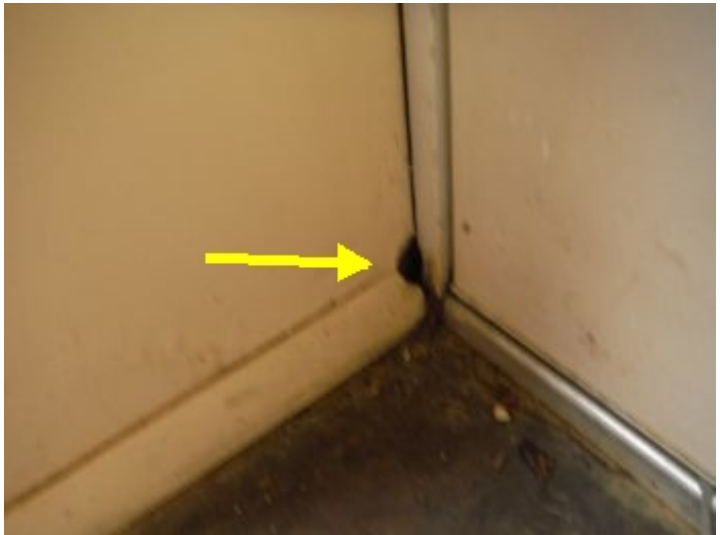
Seal all gaps/openings / Pest hole
