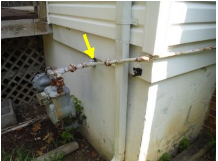
Failed or Missing sealant
