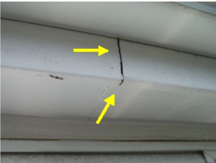
Failed or Missing sealant
