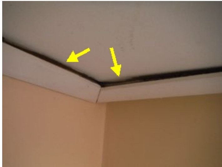
Recommend weather stripping
