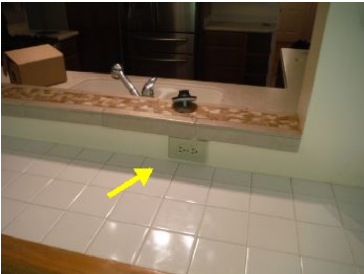
Missing GFCI protection
