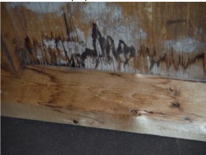
Water stains present.
