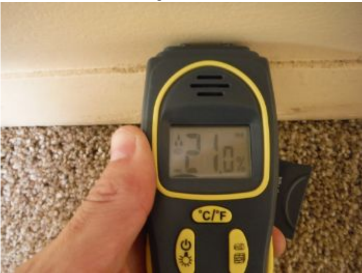
Elevated moisture reading Basement wall
