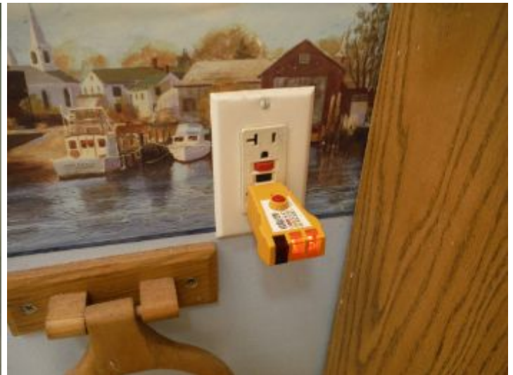
Failed or missing GFCI Basement bath
