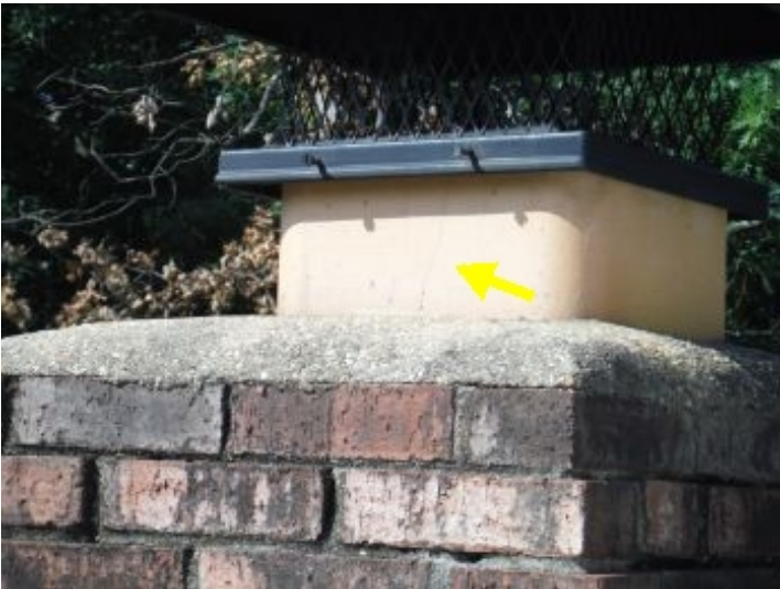
Crack in Flue tile
