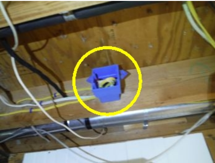
Junction Box cover missing.
