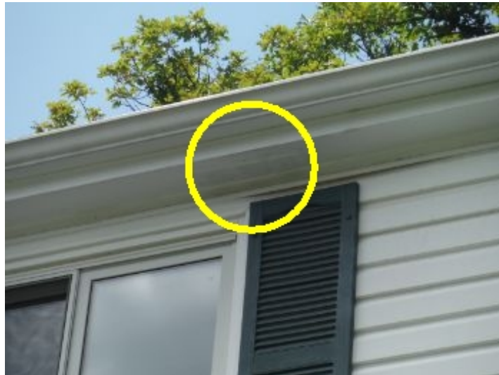
Soffit vents seem inadequate
