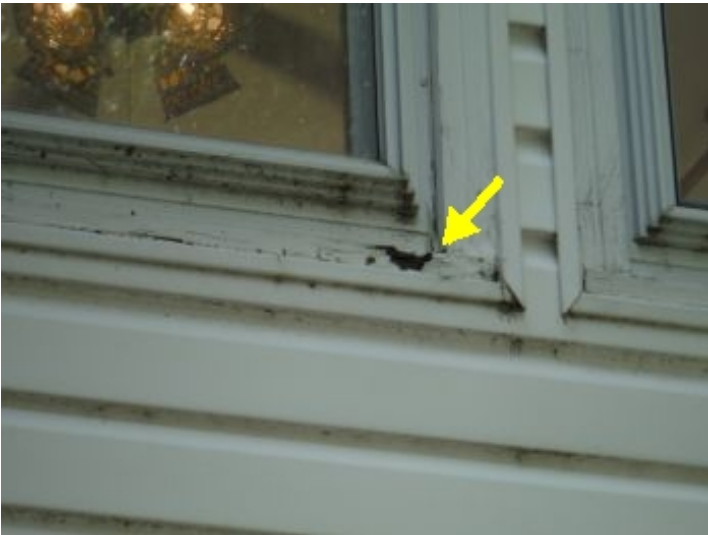
Damaged window frame.
