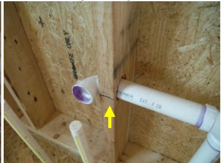
Missing nail plate
