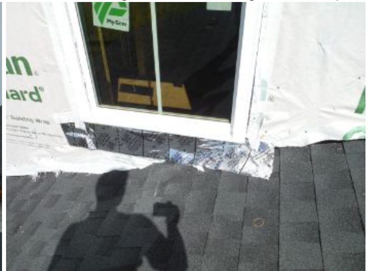
Loose, damaged and/or missing house wrap
