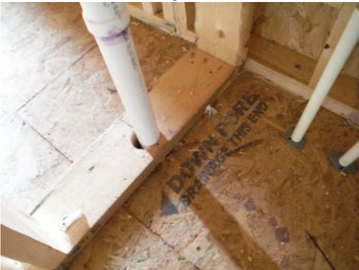
Missing nail plate
