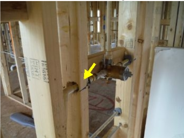
Hole to close to edge
