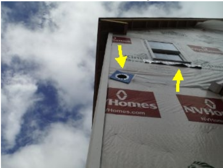
Tape loose and/or missing
