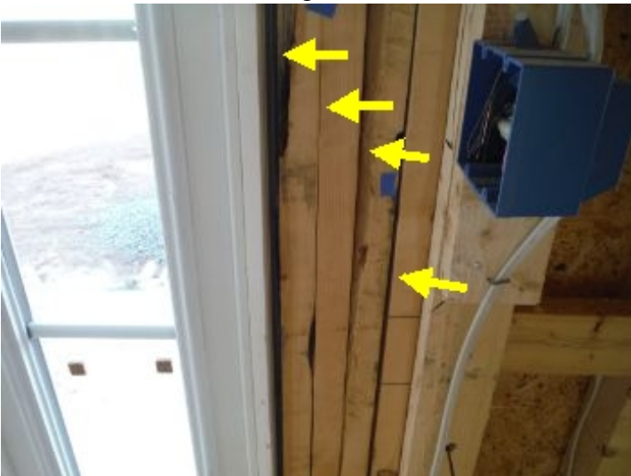
Missing sealant Front door
