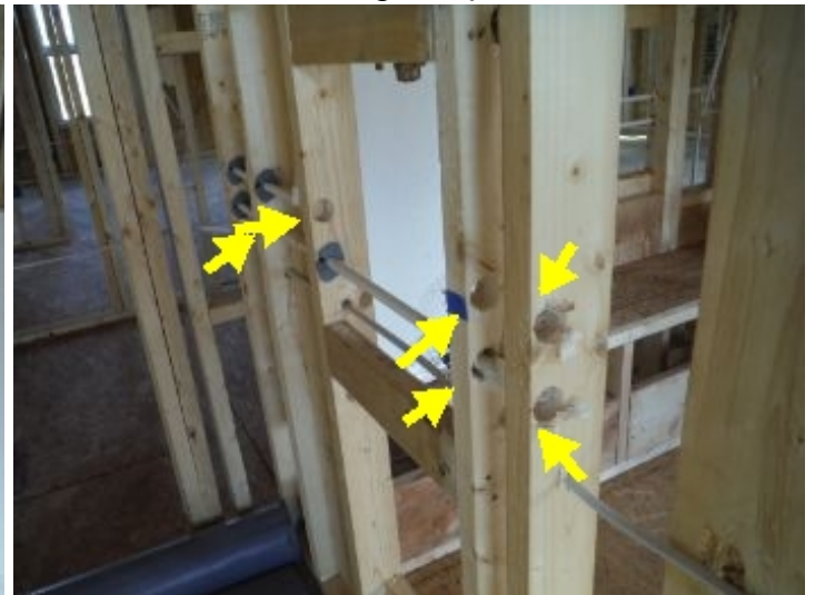
Hole to close to edge
