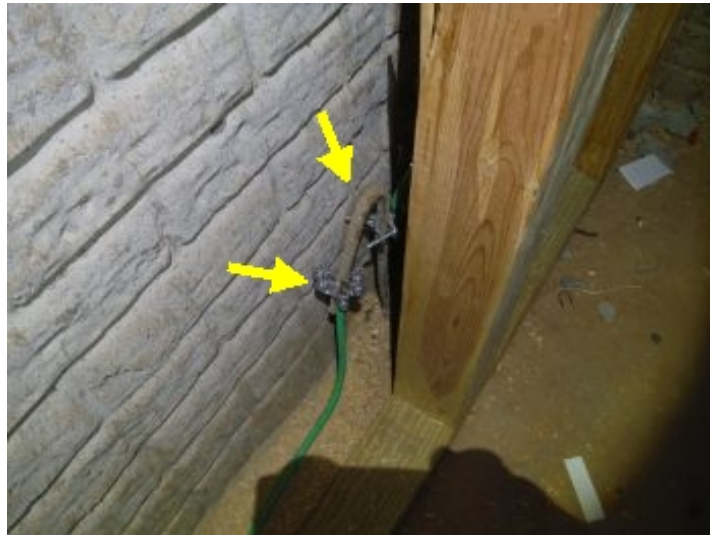
Ufer rod grounding connection
