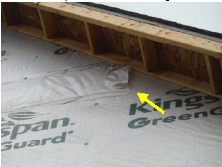
Loose, damaged and/or missing house wrap
