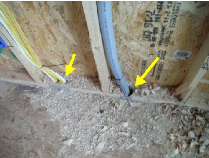
Missing fireblock Study
