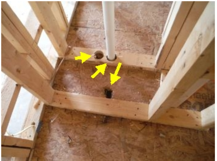
Fireblock not visible/ hole in floor sheathing
