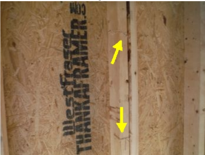
Damaged framing member
