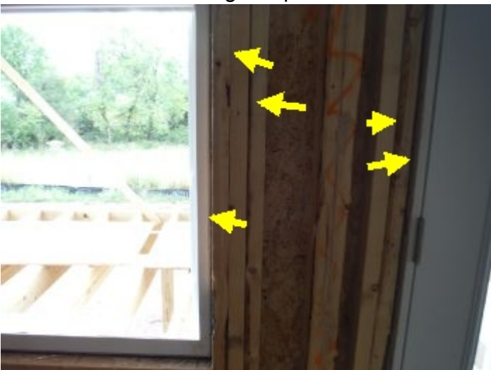
Missing sealant Living area
