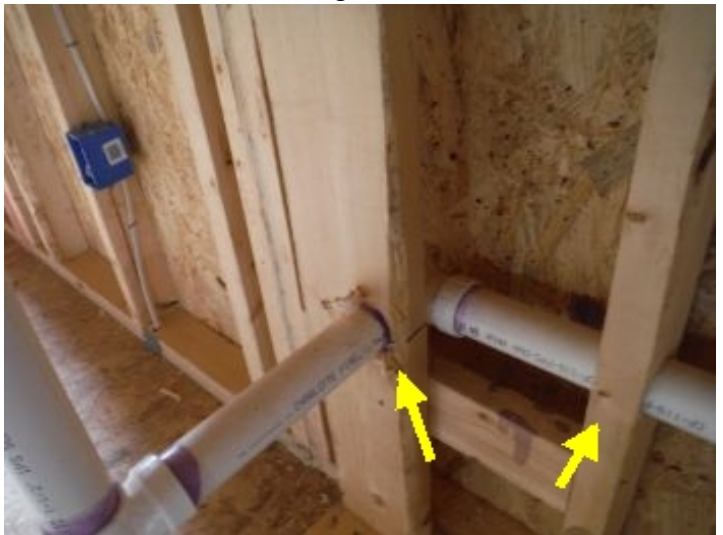
Missing nail plate Main lvl bath
