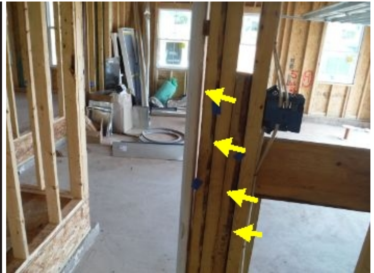
Missing sealant Garage door
