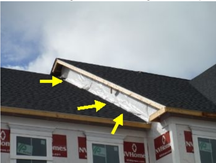
Loose, damaged and/or missing house wrap
