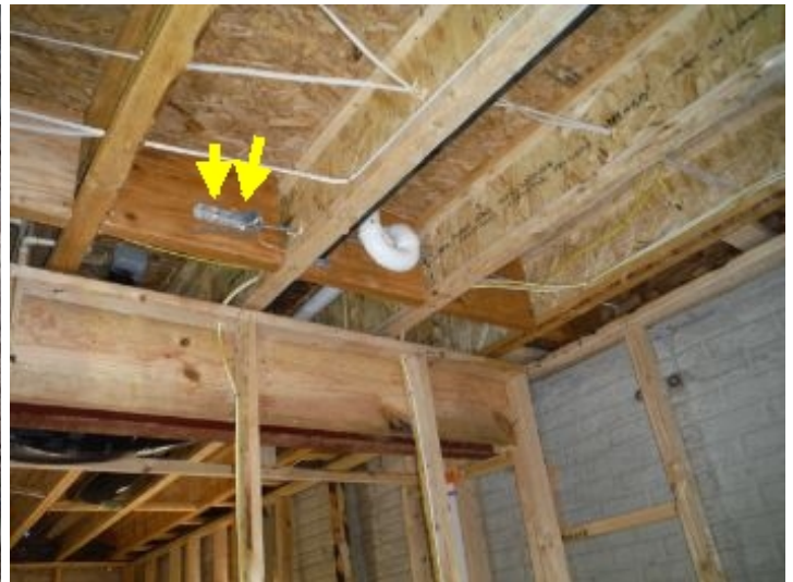
Loose and missing fastener
