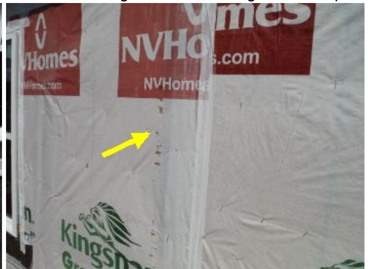
Tape loose and/or missing
