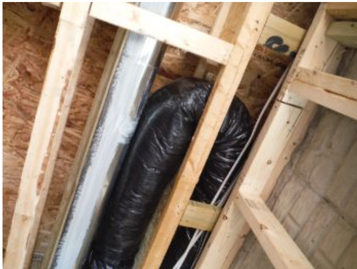
Excessive duct bend
