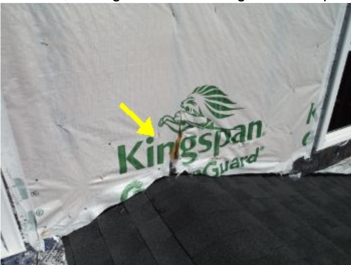
Loose, damaged and/or missing house wrap
