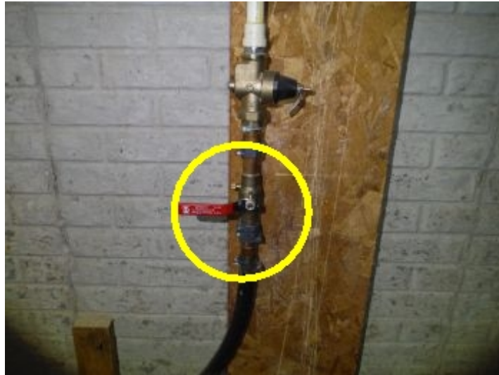
Main supply shut off
