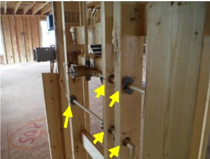
Missing nail plate
