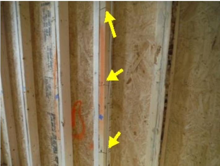
Damaged framing member
