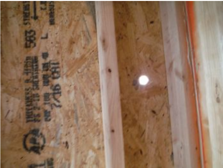
Unused hole in sheathing
