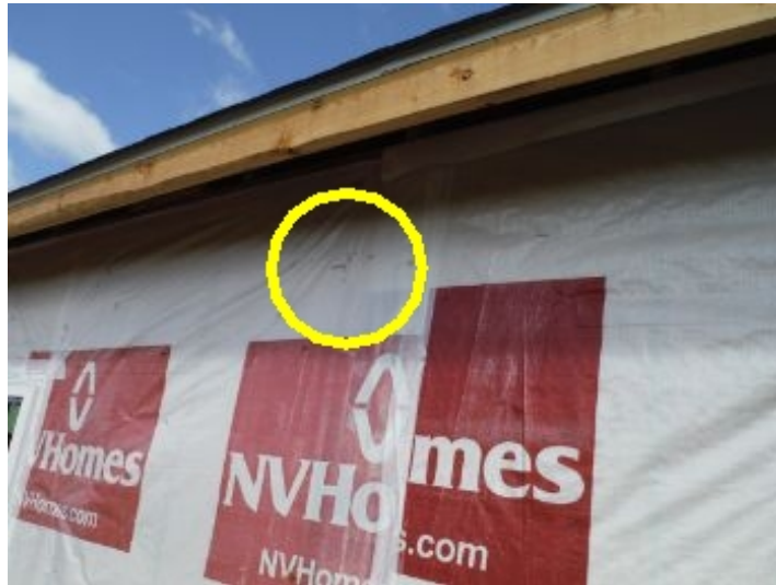
Loose, damaged and/or missing house wrap
