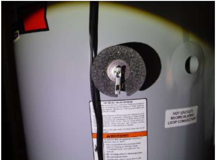
TPR valve line missing
