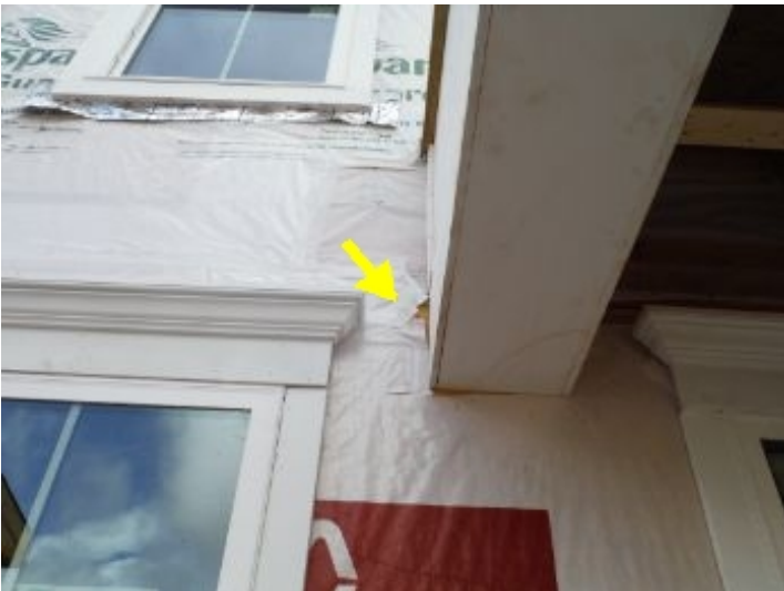
Loose, damaged and/or missing house wrap
