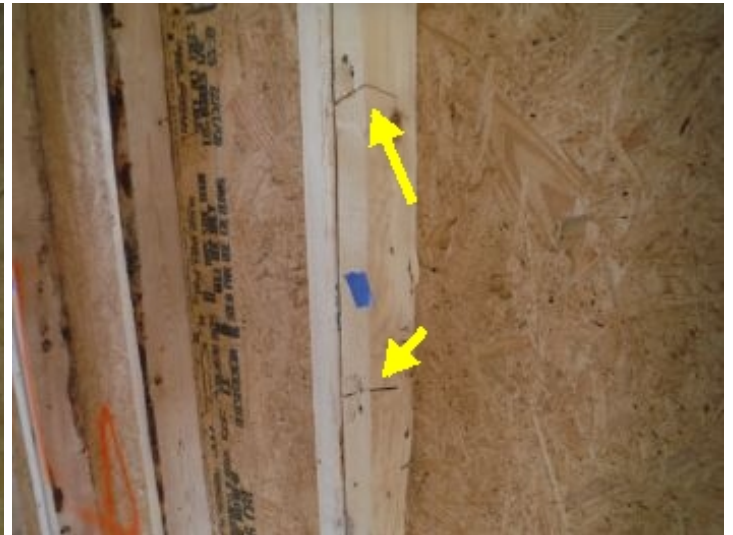
Damaged framing member
