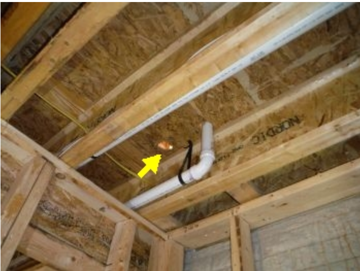
Hole in sheathing
