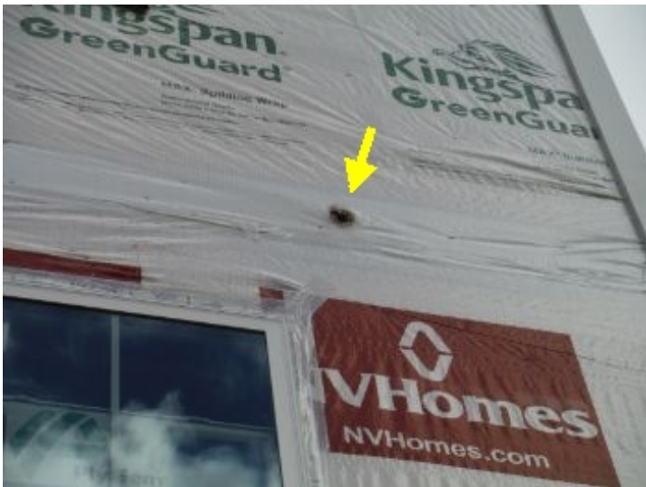
Hole in sheathing
