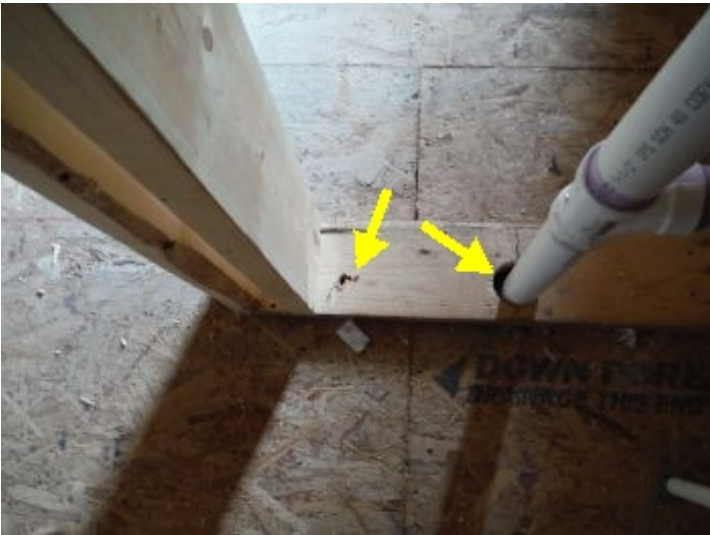
Missing fireblock Main lvl bath
