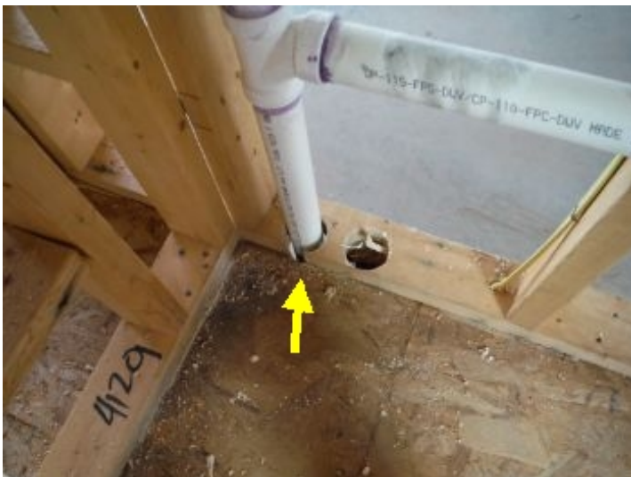
Missing nail plate
