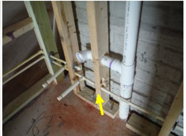
Missing nail plate
