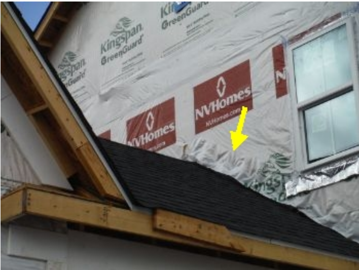
Loose, damaged and/or missing house wrap
