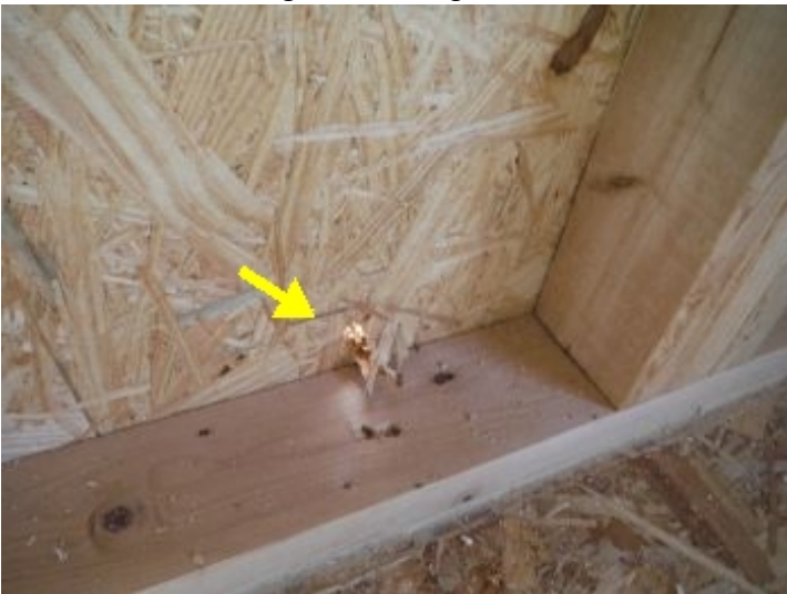
Hole in sheathing
