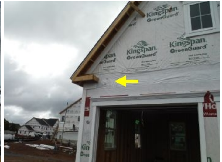
Loose, damaged and/or missing house wrap
