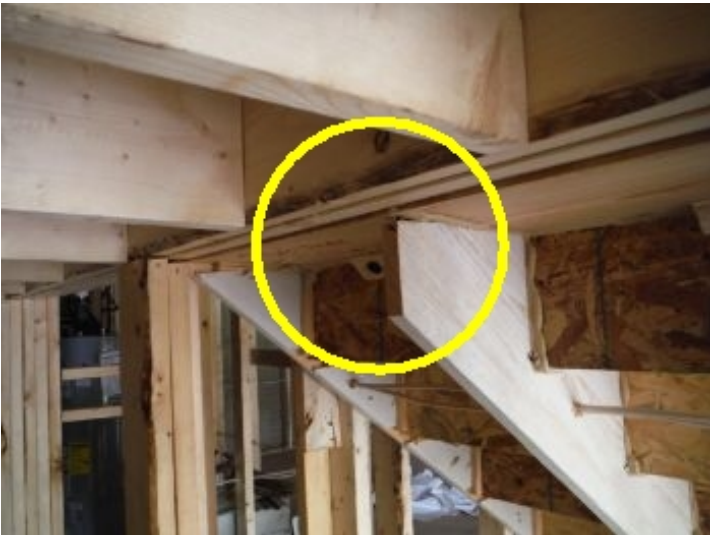
Missing bearing or hanger
