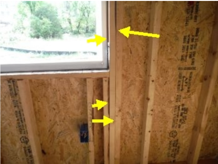
Missing sealant Laundry
