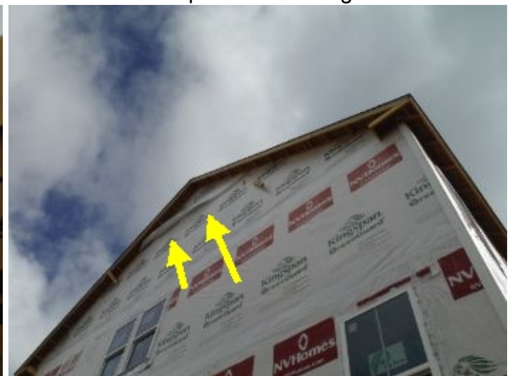
Loose, damaged and/or missing house wrap
