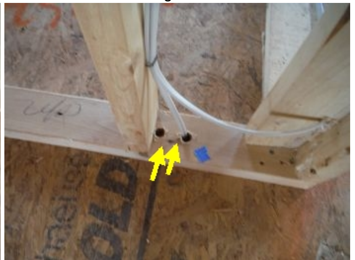
Missing fireblock Primary
