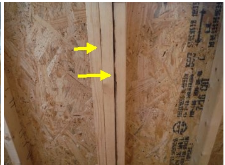
Missing sealant Laundry
