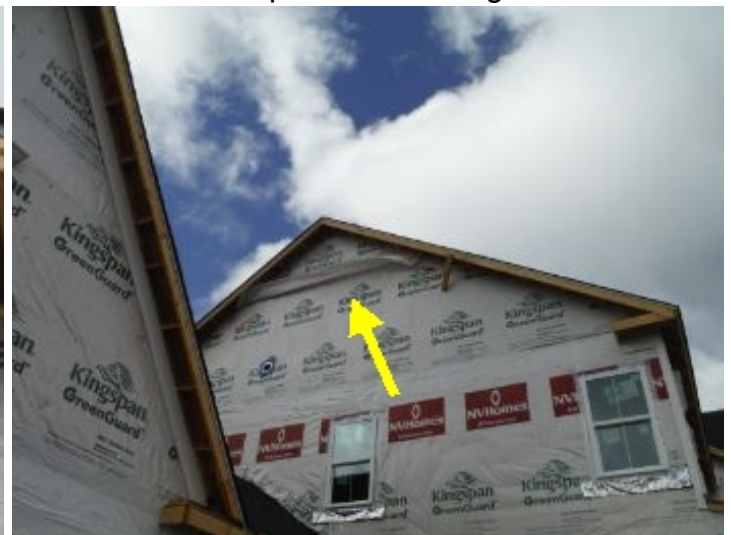
Loose, damaged and/or missing house wrap
