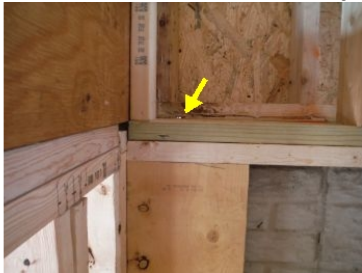
Missing sealant Stairs
