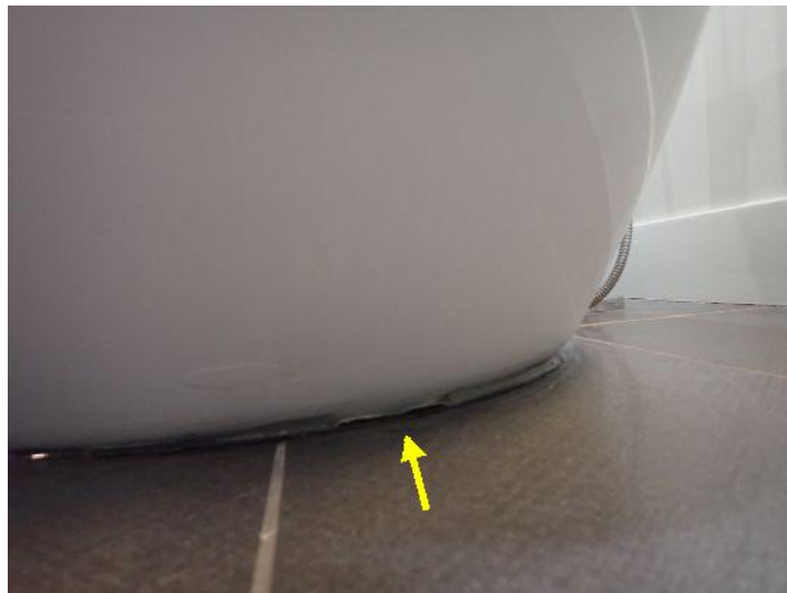
Failed and/or Missing sealant Primary bath
