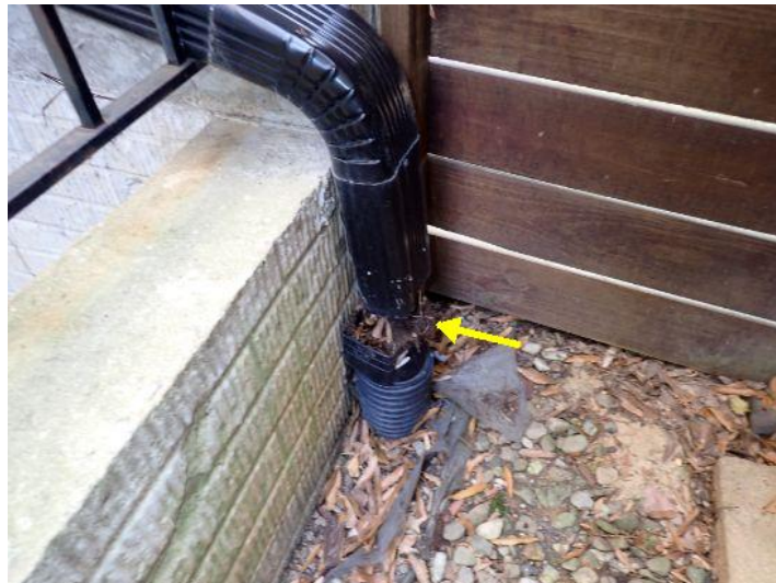
Disconnected downspout extension.
