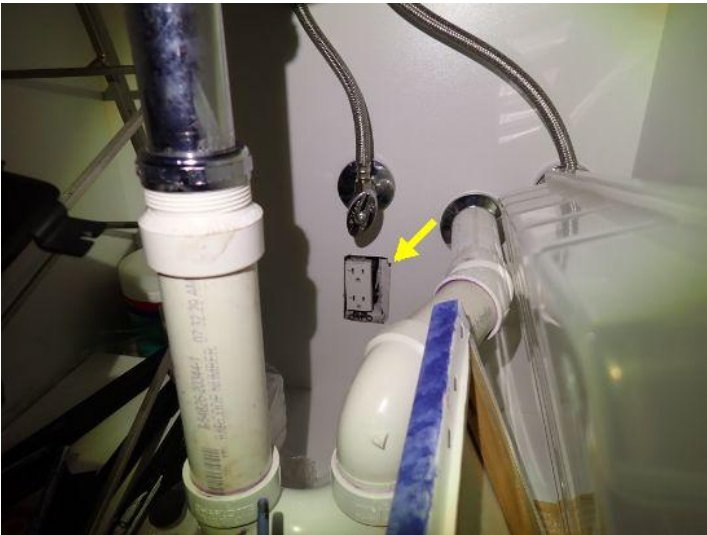
Missing receptacle cover Basement bar
