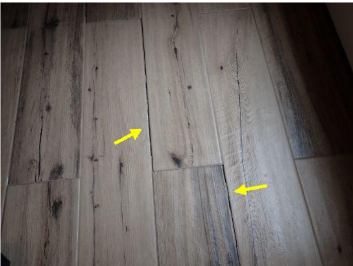
Failed and/or missing sealant Basement walkout
