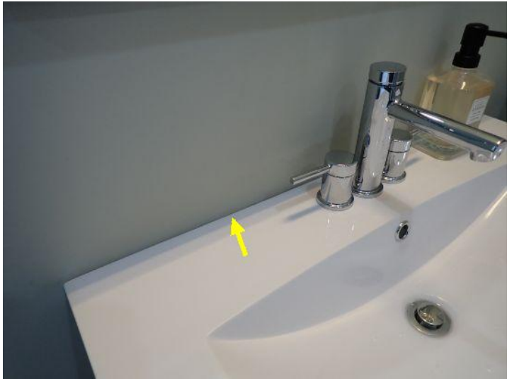
Failed and/or Missing sealant Primary bath
