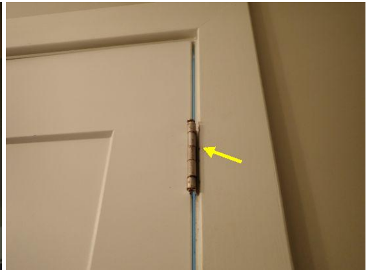
Rusted hardware J&J bath
