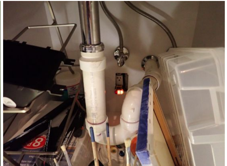
Failed or missing GFCI Basement bar
