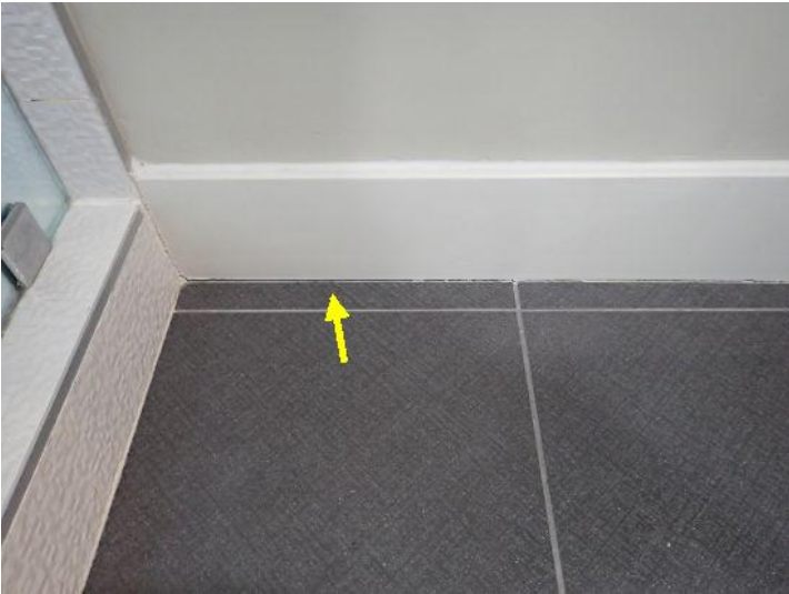
Failed and/or Missing sealant Primary bath
