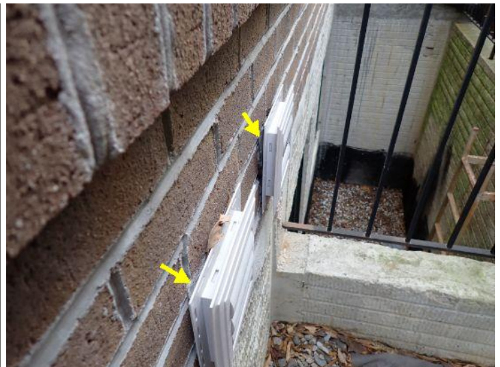
Failed or Missing sealant
