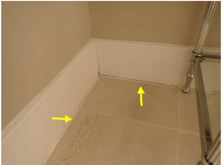
Failed and/or Missing sealant Basement on suit bath
