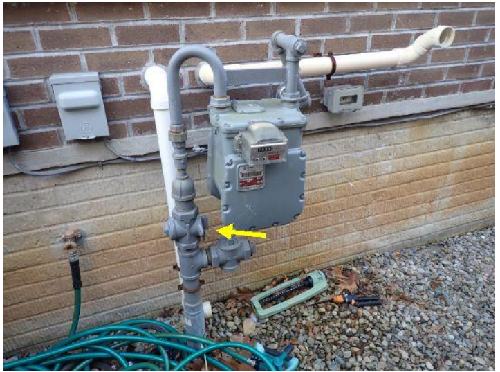
Main Gas shut off.
