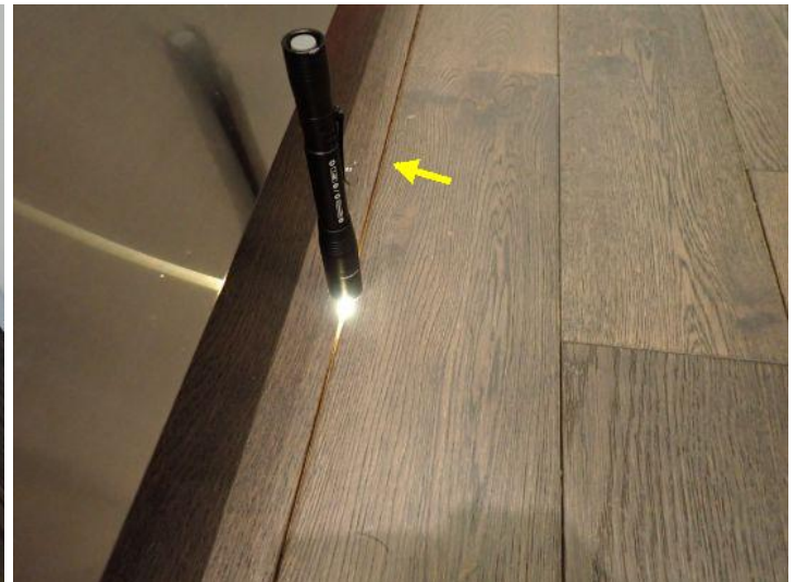
Gap in flooring
