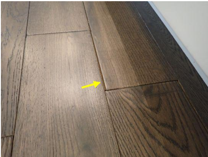
Gap in flooring
