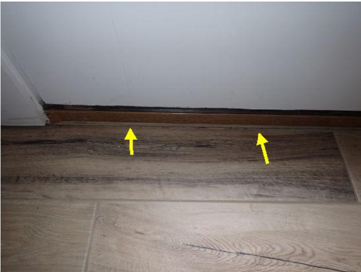
Failed and/or missing sealant walkout Basement
