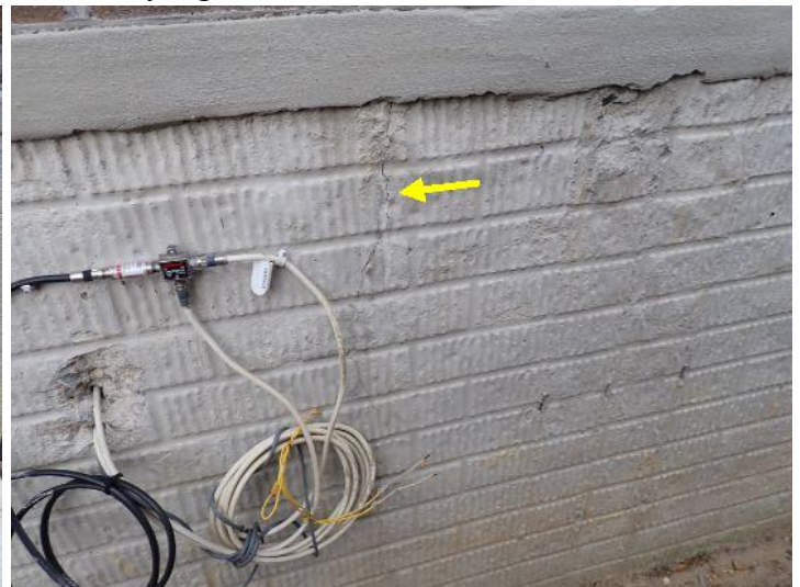
Crack visible Left side
