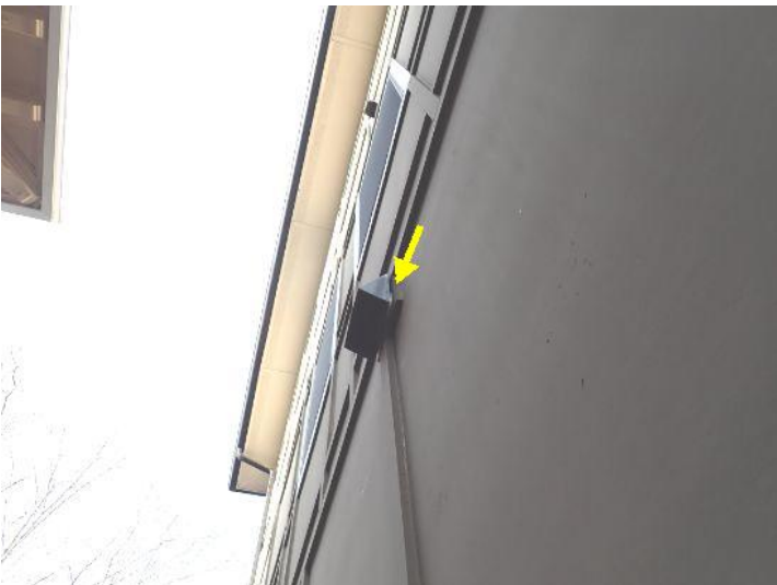
Failed or Missing sealant
