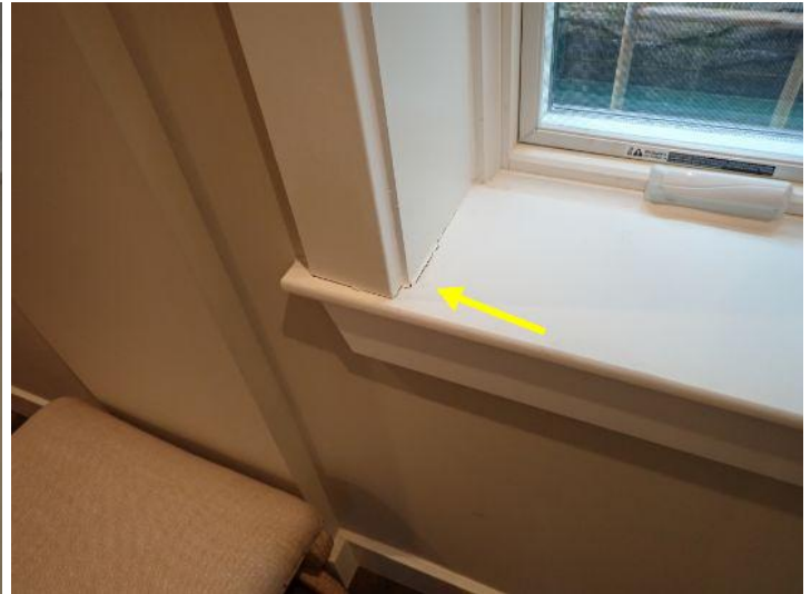
Failed and/or Missing sealant
