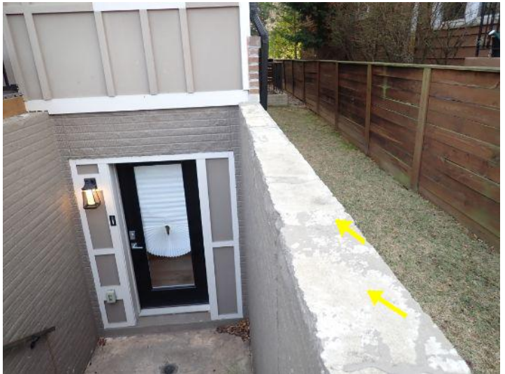
Failed or missing paint
