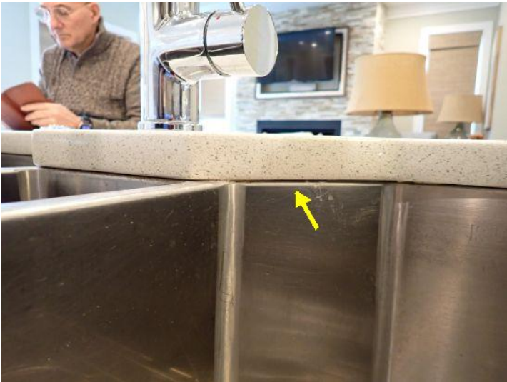
Failed or missing sealant
