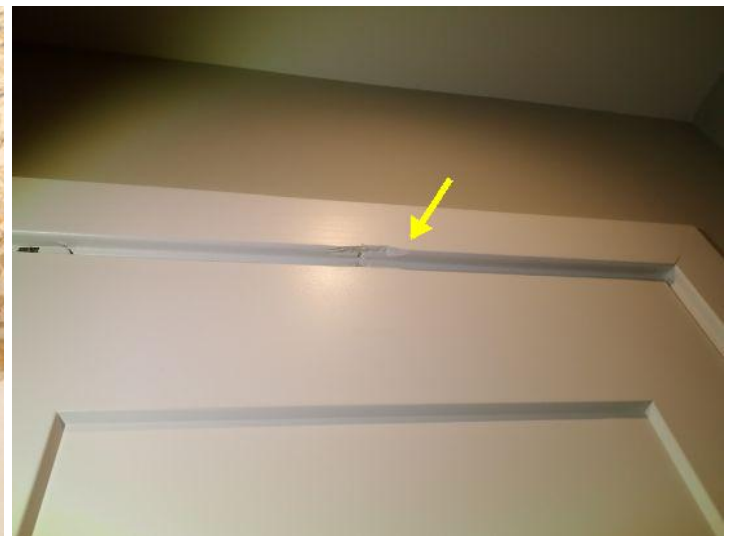
Damaged trim. Basement bedroom
