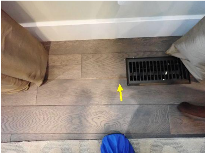
Gap in flooring
