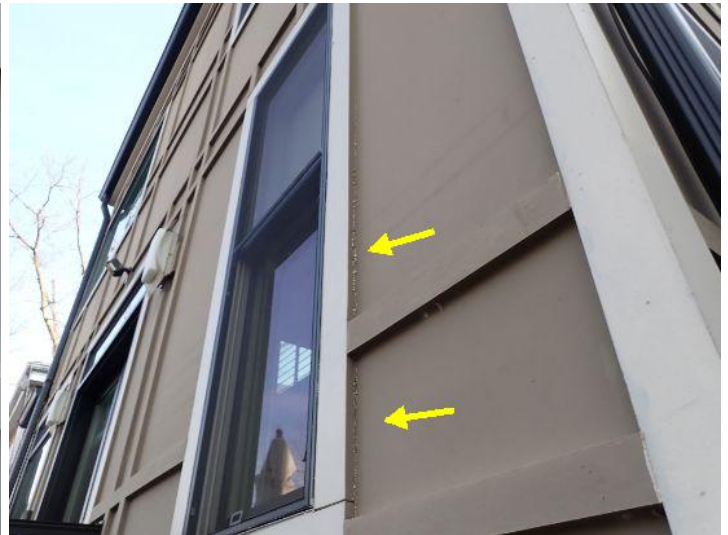
Failed or Missing sealant Rear
