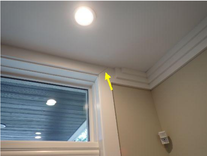
Failed and/or Missing sealant
