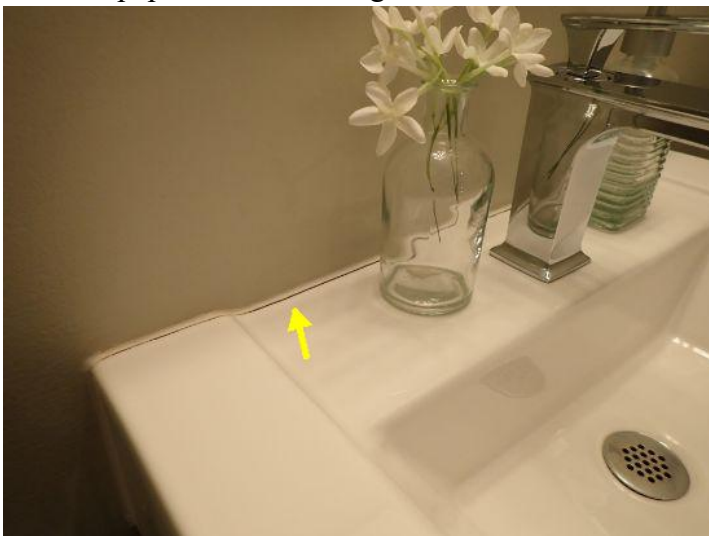
Failed and/or Missing sealant Half bath
