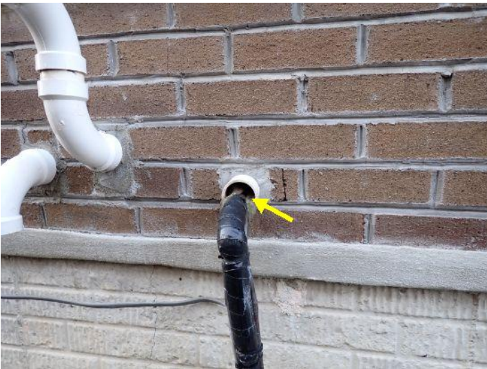
Failed or Missing sealant
