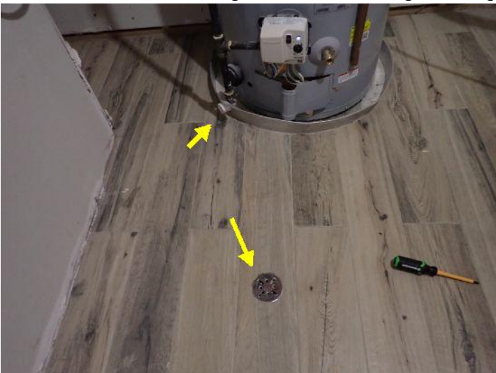
Missing drain line
