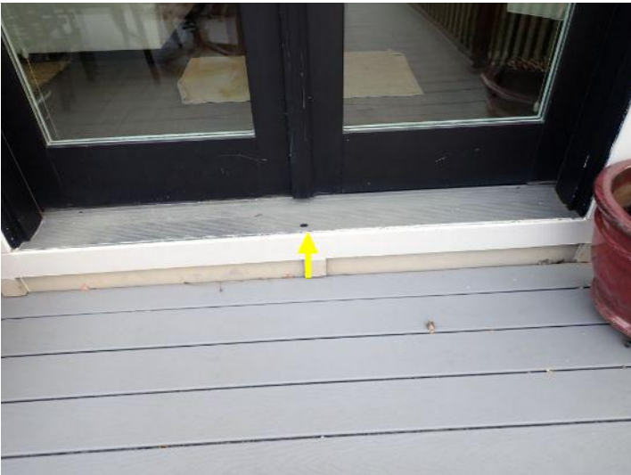
Failed or missing sealant
