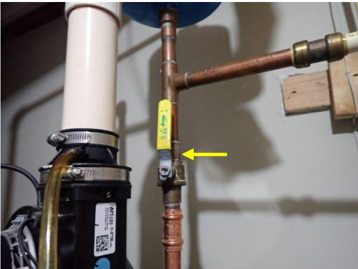
Water heater supply shut off.
