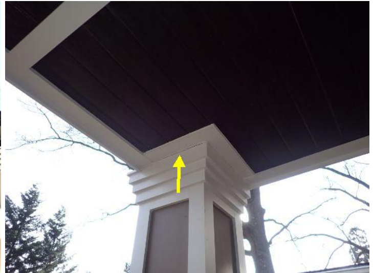
Failed or Missing sealant
