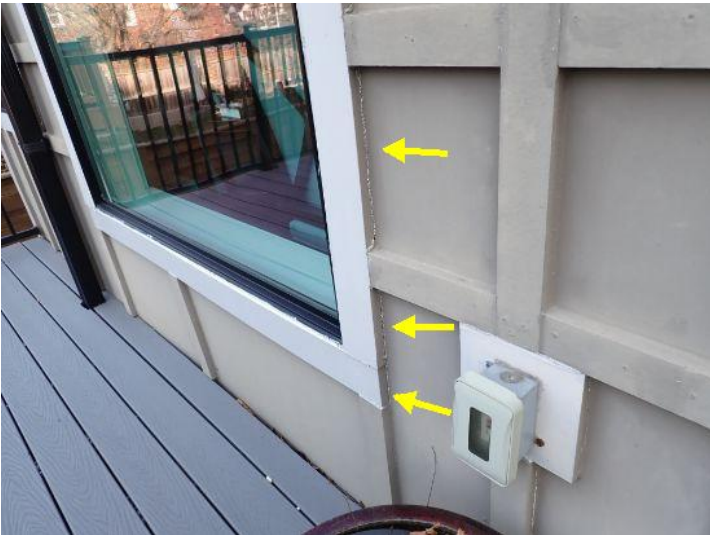
Failed or Missing sealant
