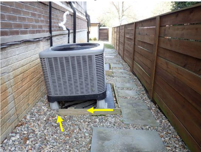
Pad not level.
