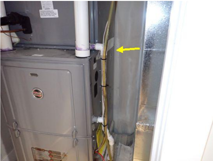
Missing "P" trap
