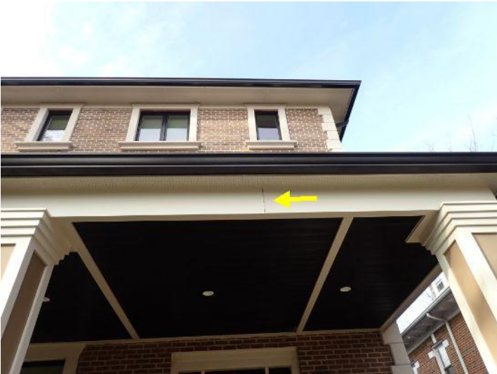
Failed or Missing sealant
