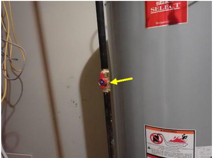
Gas supply shut off. Water Heater
