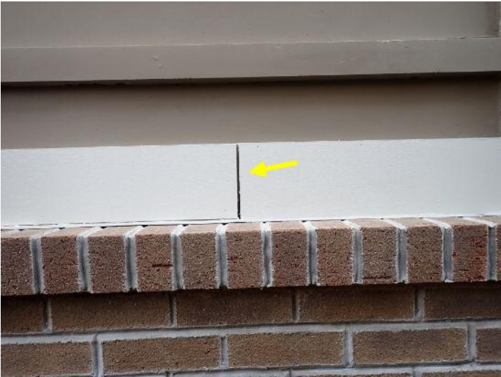
Failed or Missing sealant
