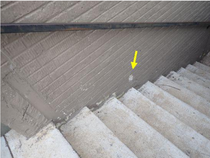
Failed or missing paint
