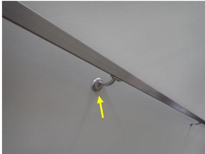
Handrail loose 3rd level
