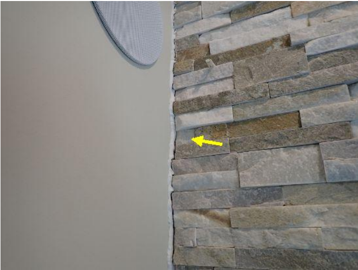
Failed and/or missing sealant Fireplace wall junction
