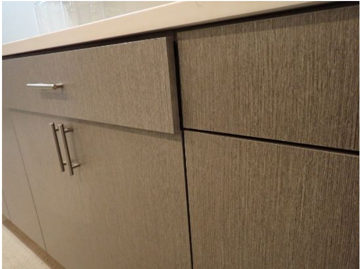
Cabinet/Drawer door misaligned Basement bar
