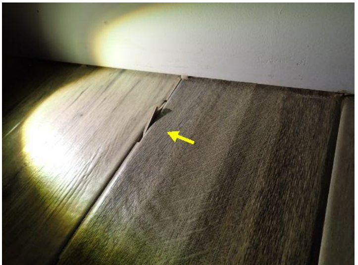
Failed and/or missing sealant Basement walkout
