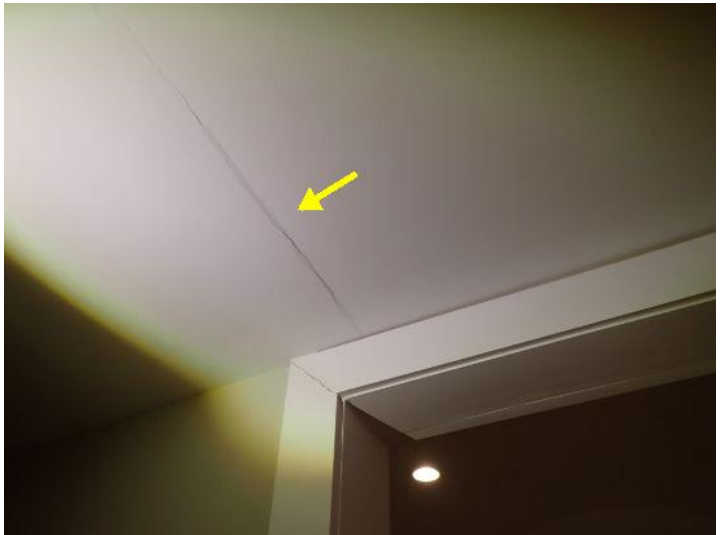
Crack in drywall Basement
