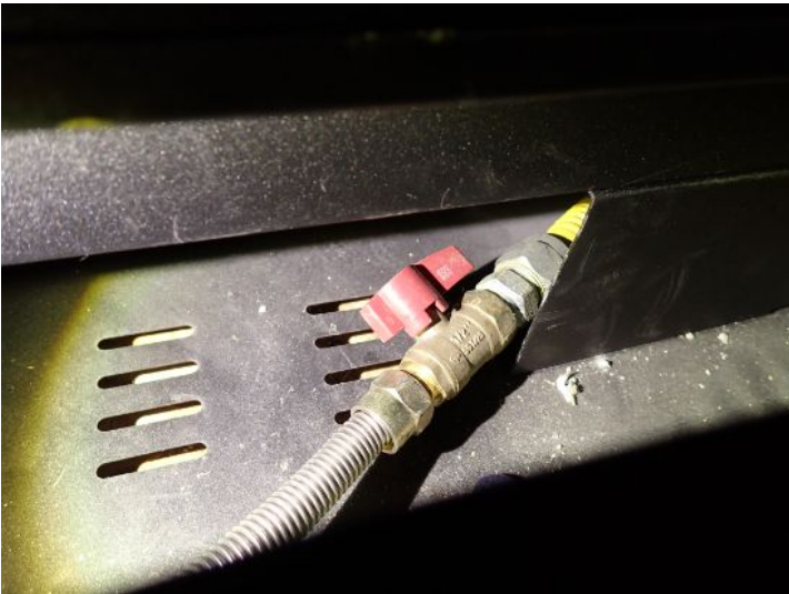
Gas supply shut off Fireplace
