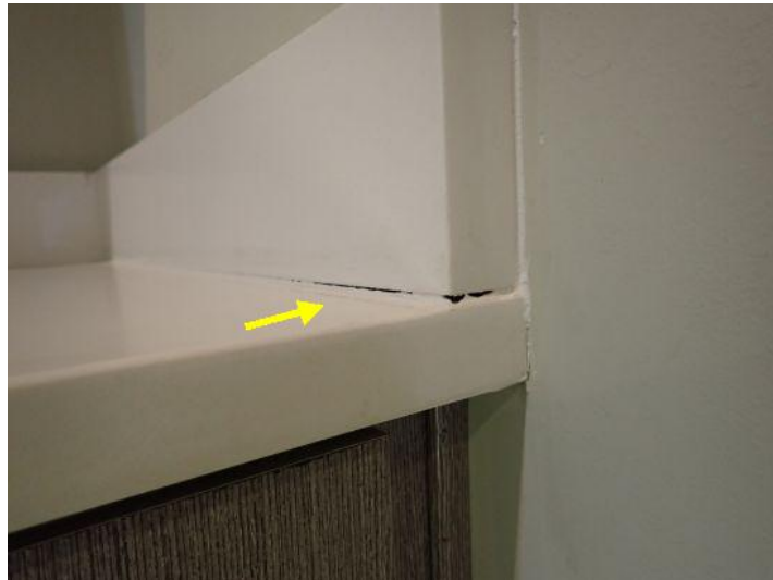
Failed or missing sealant Basement bar
