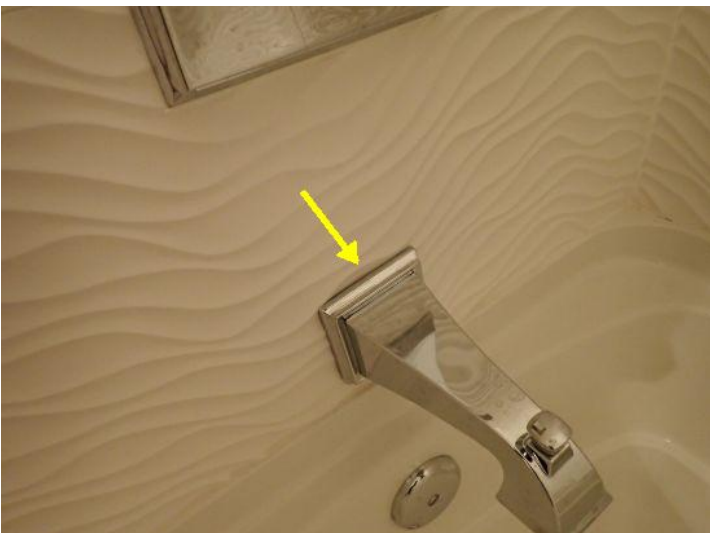
Failed and/or Missing sealant J&J bath
