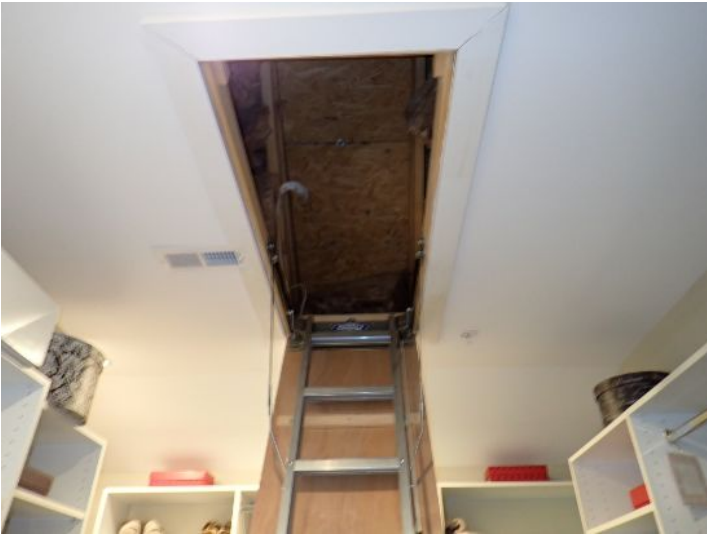
No insulation over attic stairs
