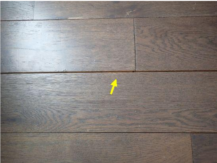
Gap in flooring
