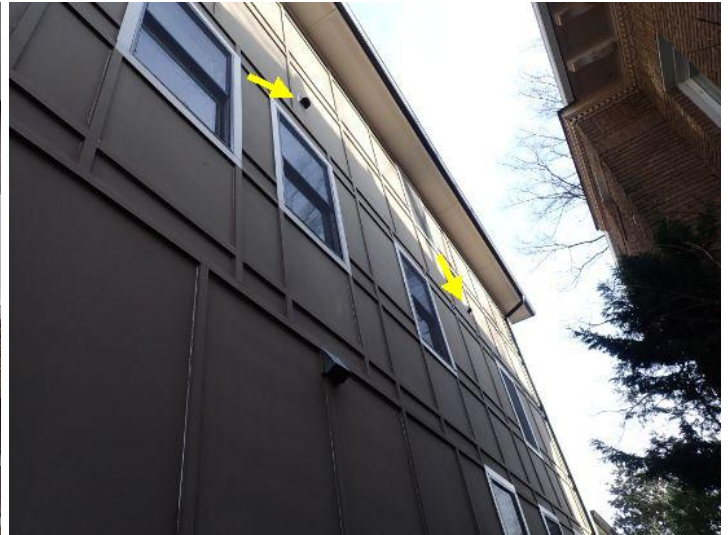
Penetration block missing/not visible
